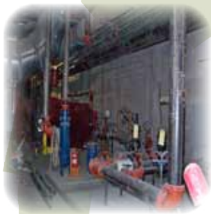
Jack Johnstone Snake Plumbing and Heating - Leask, Sask.
